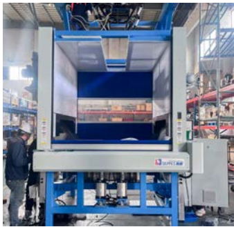
Customized inverted installation structure
