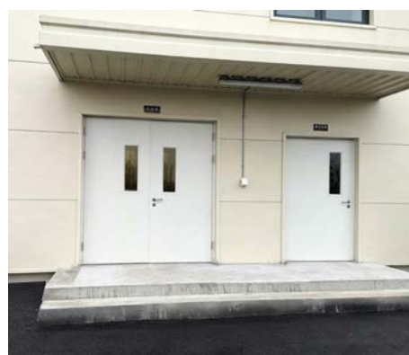
Steel Fire-Rated Door
