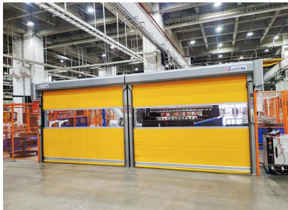
Robot Equipment Fence
