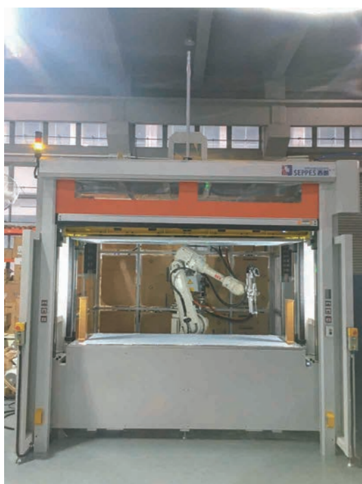
Robot Workshop Protective Door
