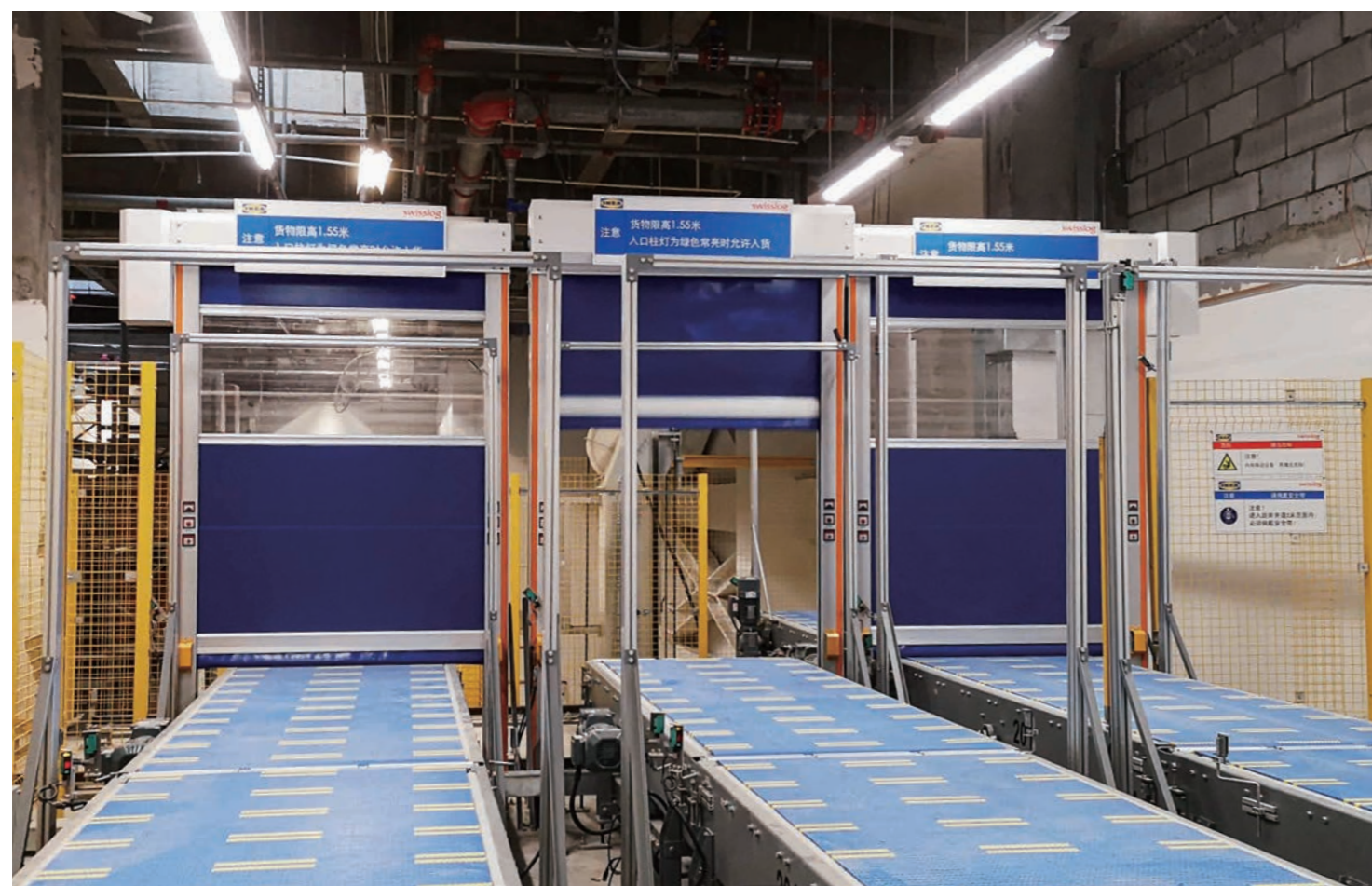
Conveyor belt linked high speed door (IKEA)
