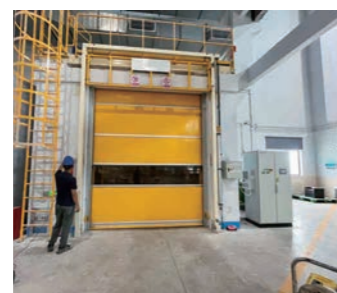
Freight elevator interlocked high speed door
