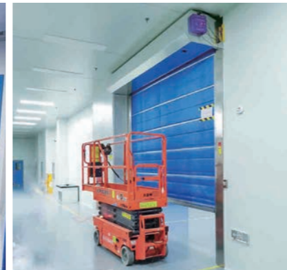
Inorganic cloth fire doors in clean areas
